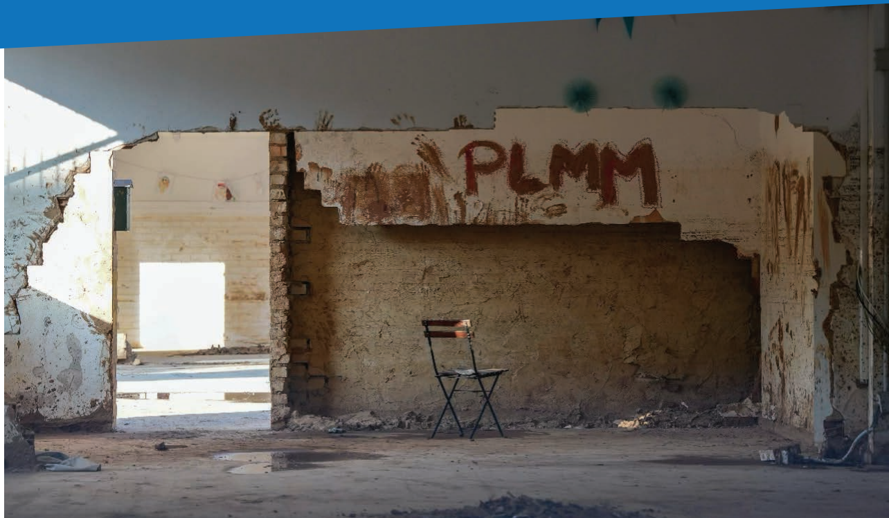
Valencia Spain, Destroyed school, DANA Floods. © Educo
