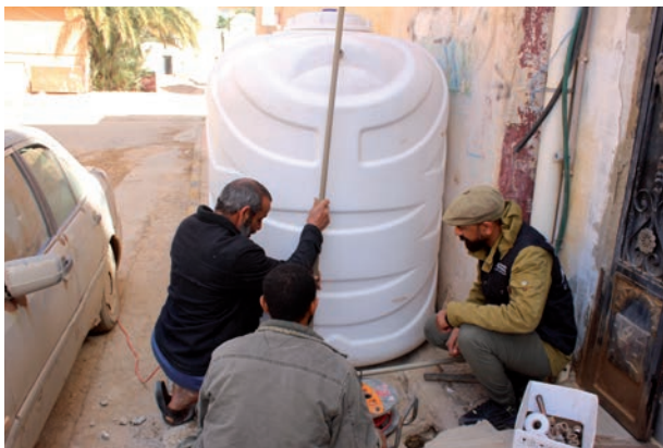
IMC staff members install the water tank near Ahmed’s house in February 2024.
